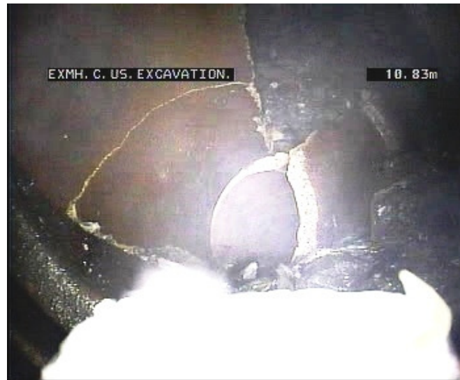
Extent of damage to pipe prior to remedial works.
