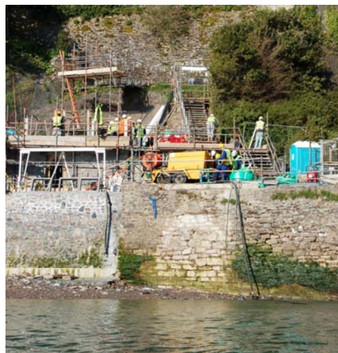
South Town Pump Station, Dartmouth.z
