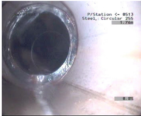
Leak prior to sealing
